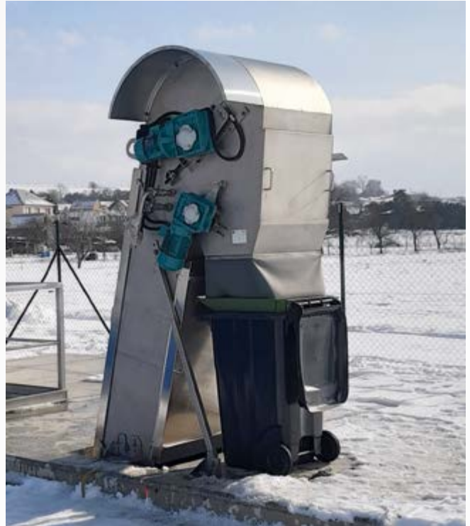
Pumping station, Sazovice, Czech Republic, 1000_CP_3250_Z
