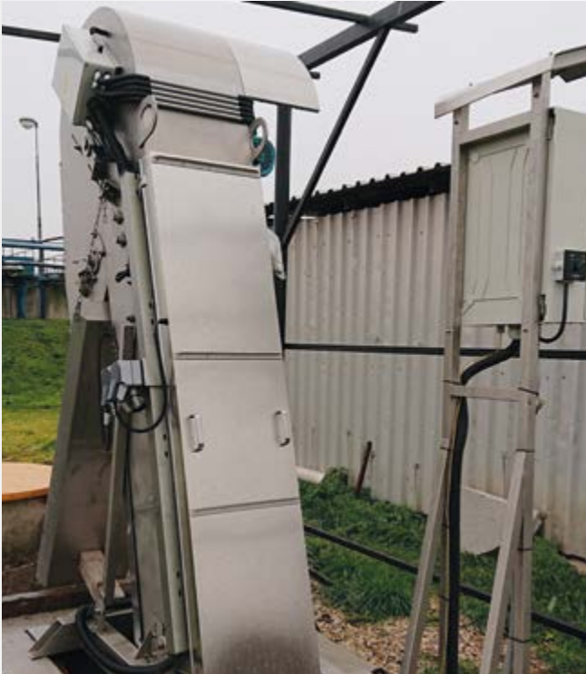
WWTP, Mojmírovce, Slovakia, 500_CP_3500_Z
