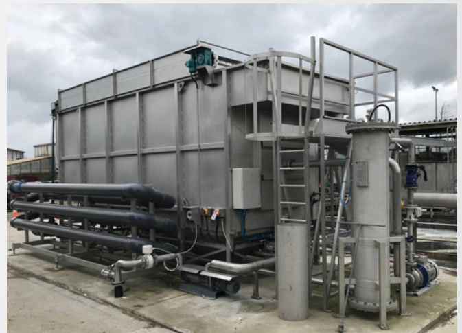
Application sample – Tannery plant, Waitoa, New Zealand, FH_100
