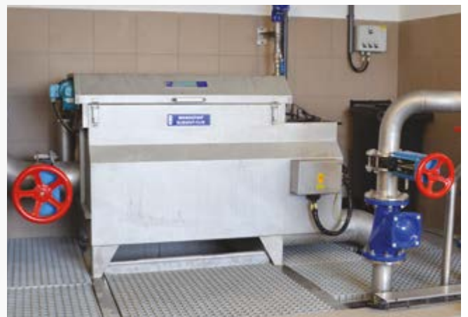
WWTP, Czech Republic, 2FBO
