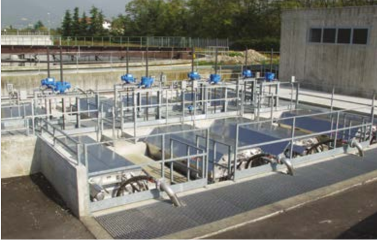
WWTP, Italy, 6FBB
