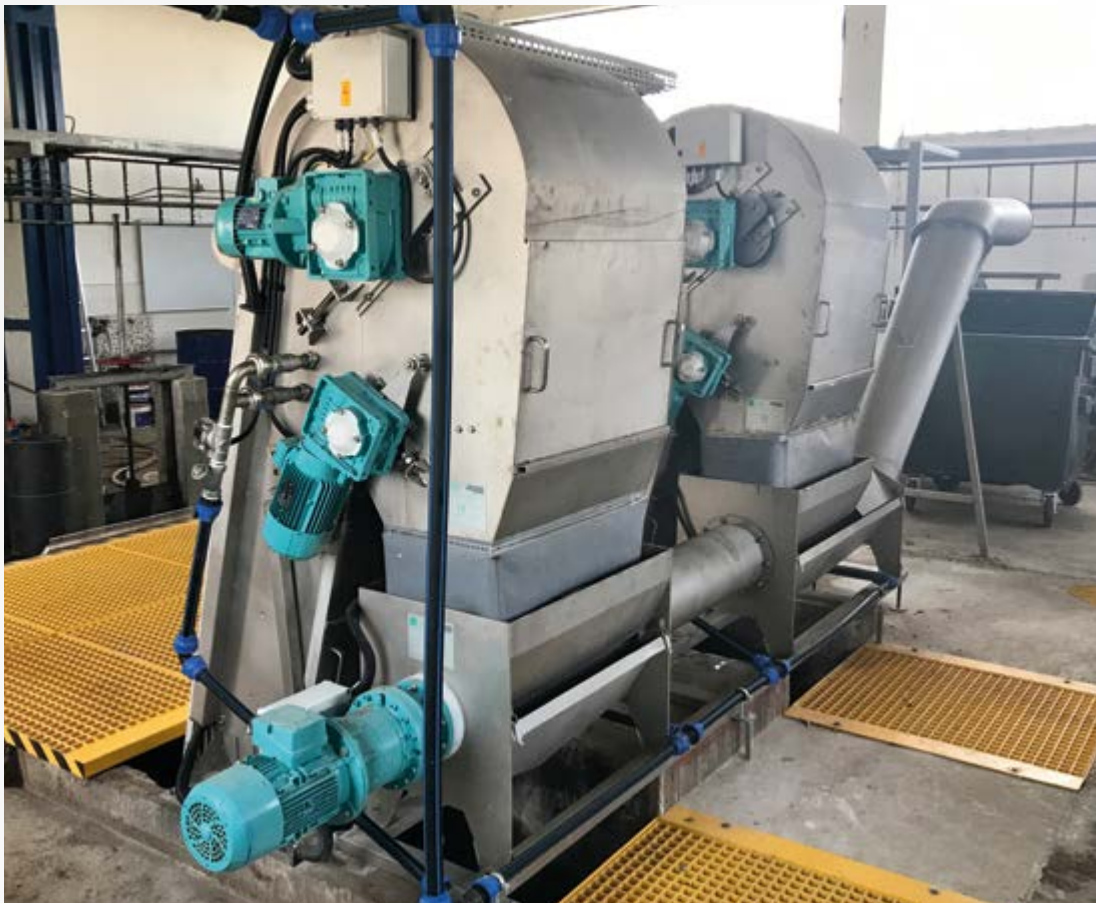
WWTP, Stupava, Czech Republic, 800_CP_1050 + LS_2400
