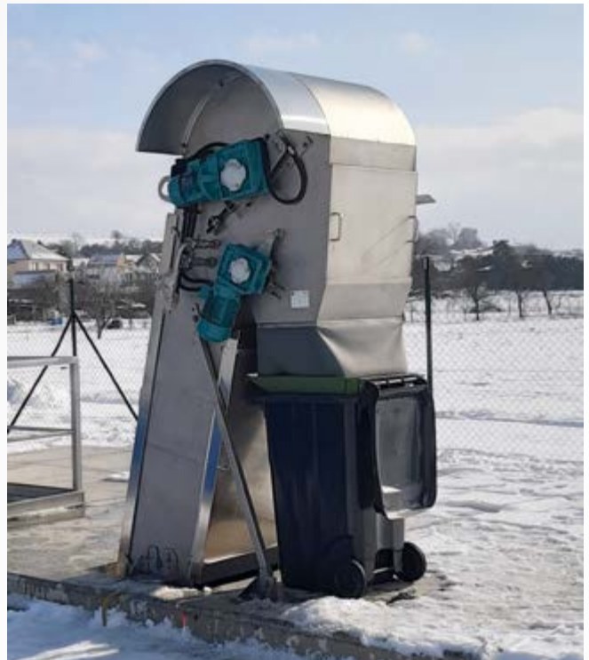
Pumping station, Sazovice, Czech Republic, 1000_CP_3250_Z
