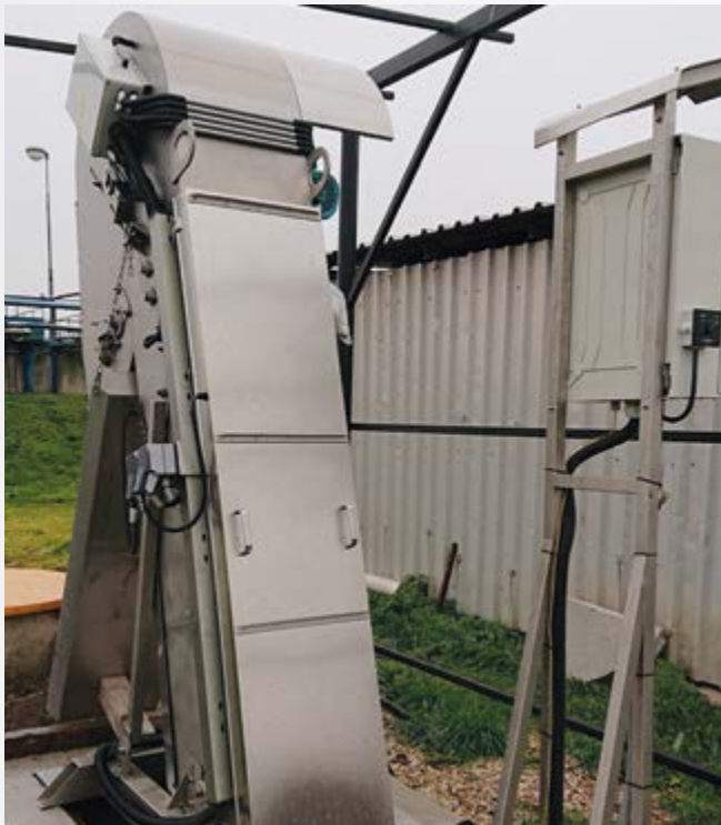
WWTP, Mojmírovce, Slovakia, 500_CP_3500_Z
