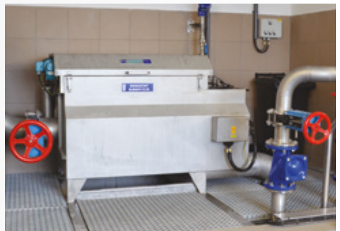
WWTP Chromeč, Czech Republic, 2FBO
